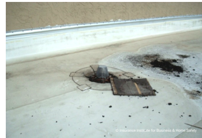
Example 3. Interior roof drain blocked by leaves and a piece of wood left behind by a contractor.
