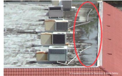
Example 4. Improperly sloped insulations boards and HVAC drain lines not funneled to drains contribute to long-term standing water.
