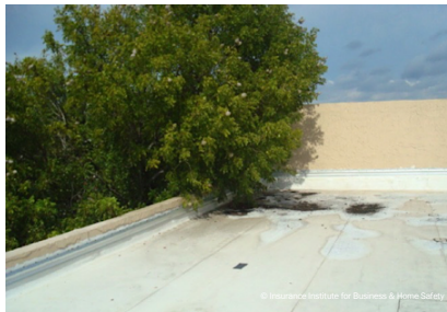
Example 2. Poor tree maintenance allowing leaves and twigs to clog roof drains.
