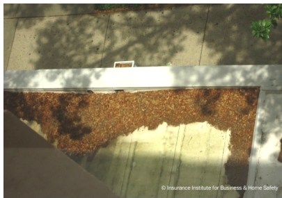
Example 1. Scupper and downspout clogged with leaves.
