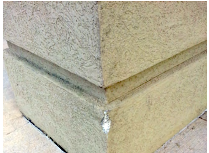
Chipped EIFS with exposed EPS at a hotel entrance near an outdoor smoking area.
