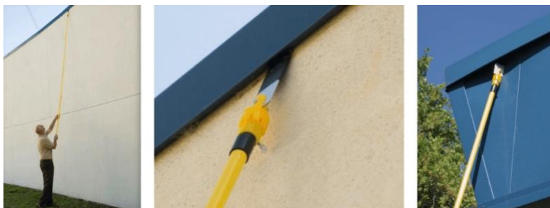
Loose or ill-fitted flashing can cause roof cover failure and water intrusion during high-wind events.
