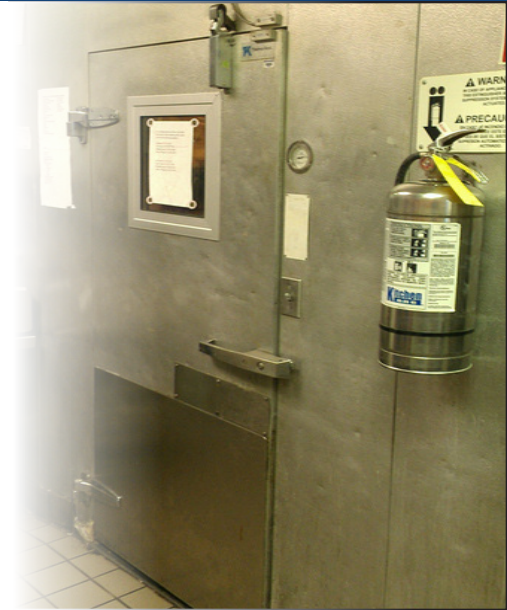
Typical walk-in cooler.
