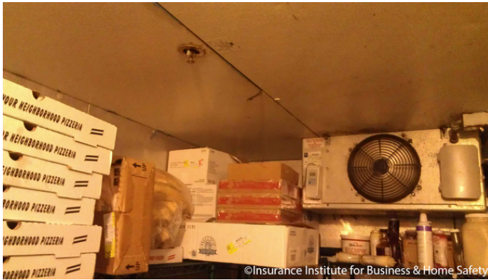
Sprinkler head located at the ceiling of this walk-in cooler.
