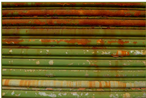
Figure 3. Inspect for rust on commercial doors. The picture above shows a severe case of rusting on a roll-up door, which can greatly decrease its strength.
