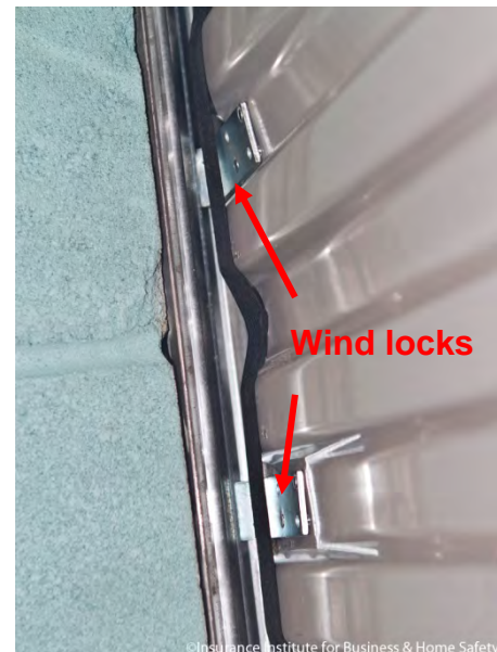
Figure 2. The roll-up door pictured above is equipped with wind locks that will keep the door from being forced out of the tracks during a windstorm.
